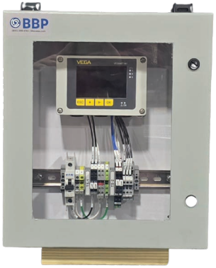
Pump Control System
