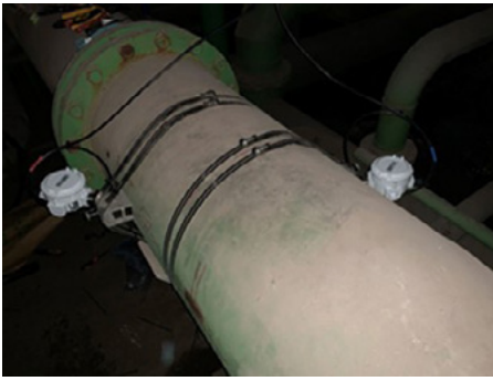
Picture 3. 50-year-old corroded pipe
