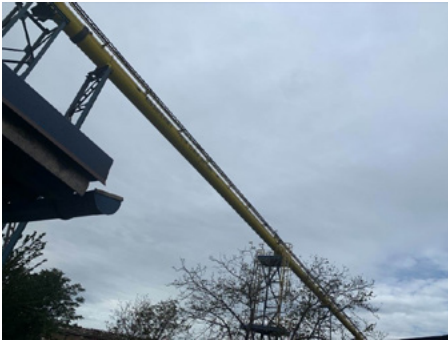
Picture 12. DN800 coke oven gas
