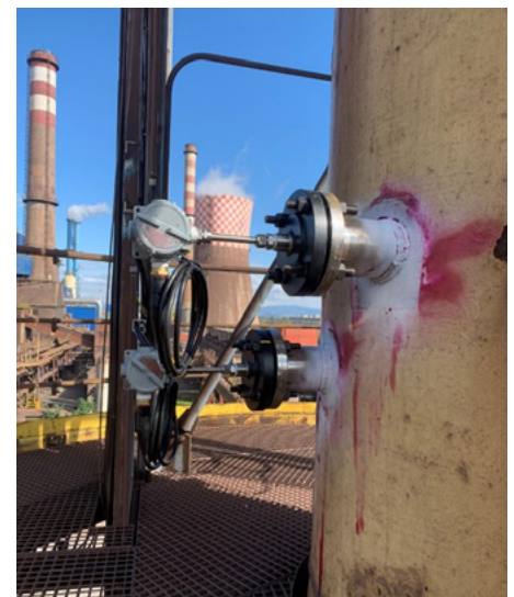
Picture 10. Combustion chimney with a T5 bias 90 setup on a DN800 (32") pipe for blast furnace gas.
